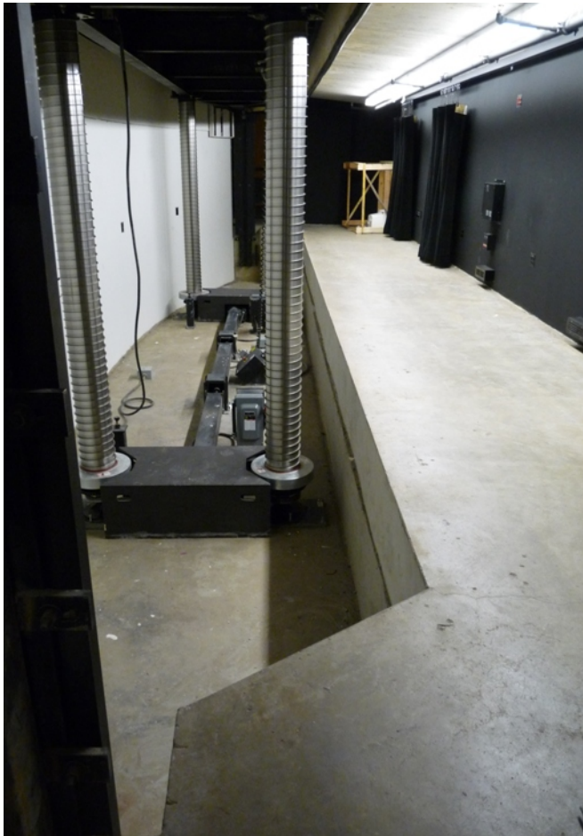
Unguarded orchestra lift machinery pit. (NOT Bolshoi New Theatre, example only) Note lack of guardrails & edge marking.
