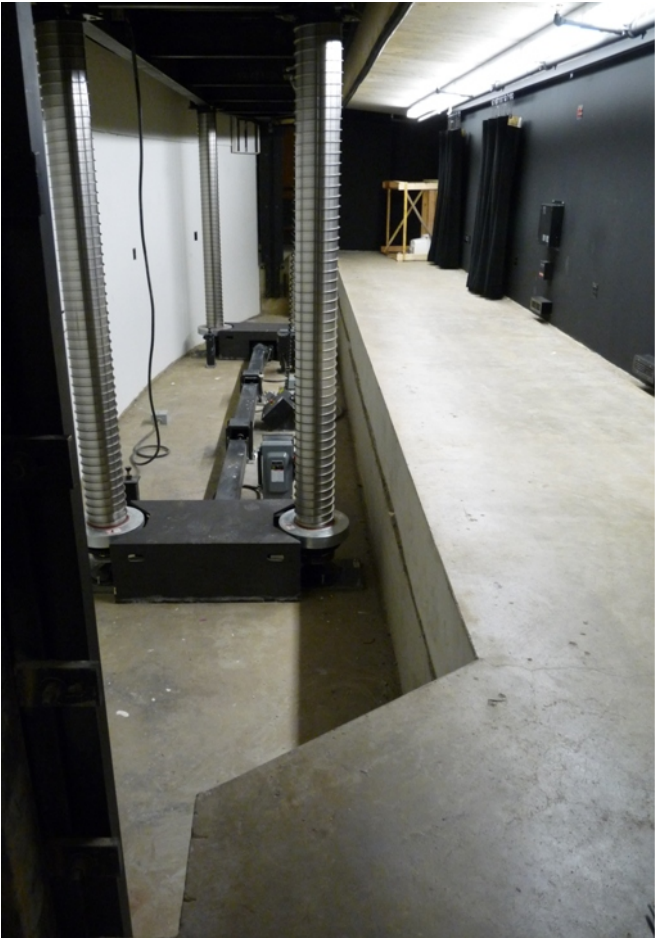
Unguarded orchestra lift machinery pit. (NOT Bolshoi New Theatre, example only) Note lack of guardrails & edge marking.
